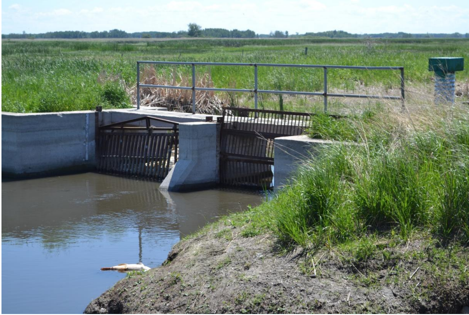
Fig 4. Screened gates at the bottom end of a channel that originates from Lake Francis (Lake Francis Outlet). Water Branch staff indicated that the dead fish were backed up against the upstream side of the gates for approximately 5 metres. Gates were opened around 10:30 am to release dead fish to Lake MB and then again around 2:00 pm. This was the site of water quality station 3. Most of the Common Carp, Freshwater Drum, White Sucker and one live Fathead Minnow were collected just upstream of the gated screen or at the crossing to the screens when the screens were opened to release the fish.
